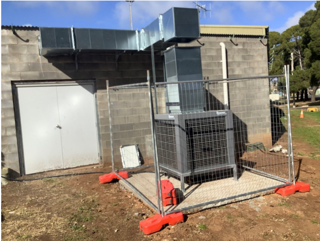
Figure 4: Ground mounted air conditioners.
